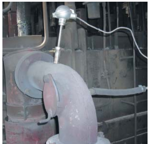
Fig. 1 Installation locations for the temperature probe sensing element and the connection of the vacuum gauge pipe
